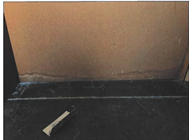
Figure 9: Visible water marking on a temporary dry wall.
