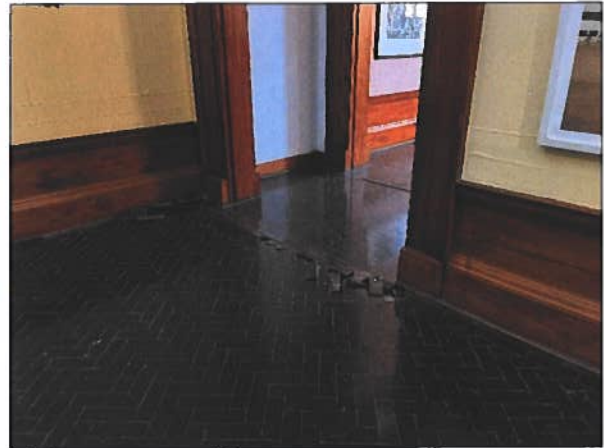
Figure 13: Lifting and loose parquet floor blocks in an exhibition hall without any caution.
