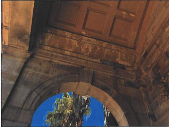
Figure 10: Visible damp at the South Entrance to the Johannesburg Art Gallery.
