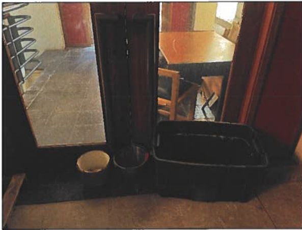
Figure 6: A temporary solution to catch incoming water, making use of buckets.
