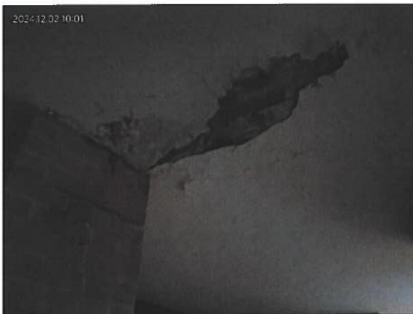
Figure 4: Blistering from water leaking has removed layers of plaster and paint.
