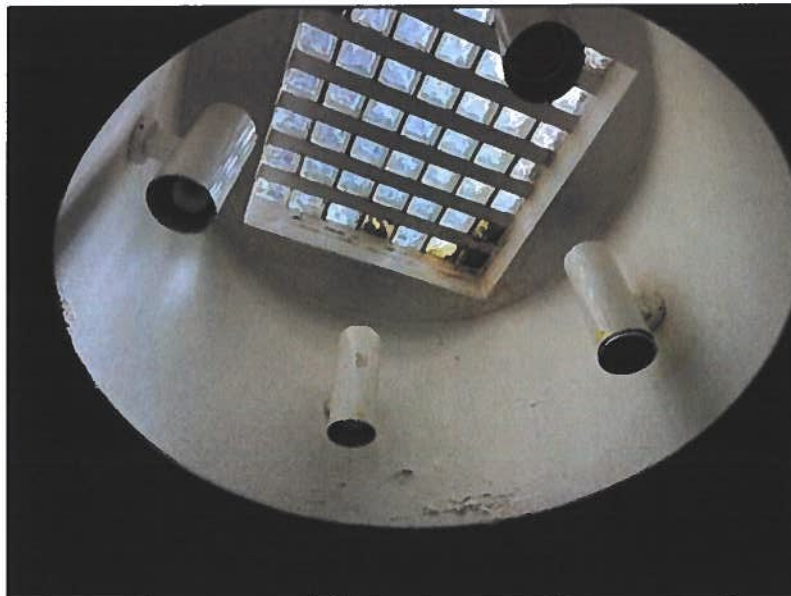
Figure 2: Blistering on masonry elements is evident, as water leaks in via gaps between glass bricks.
