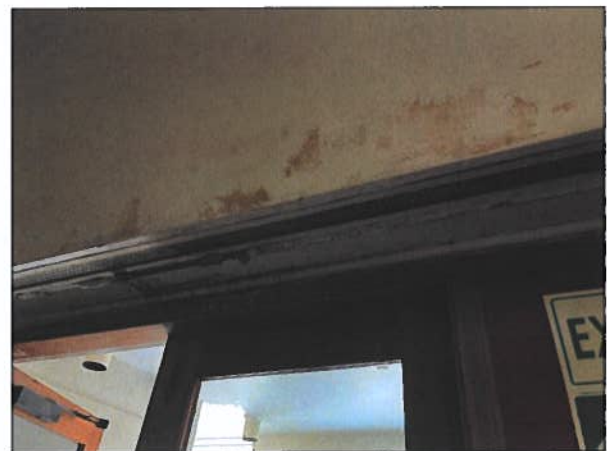
Figure 5: Water ingress visible in a storeroom at the door lintel.
