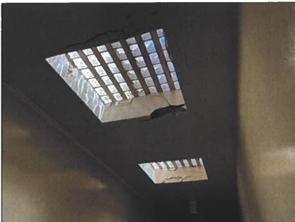
Figure 12: Imminent structural failure at a skylight.
