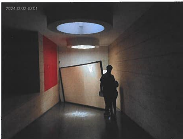
Figure 8: Looking down a sloping passage towards a storage room, with a temporary solution to prevent access.
