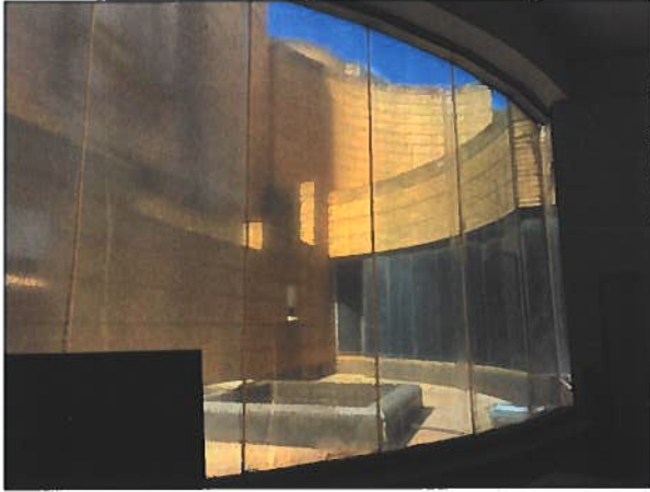
Figure 14: Poorly sealed large window sections in the Meyer Pienaar section of the Johannesburg Art Gallery.
