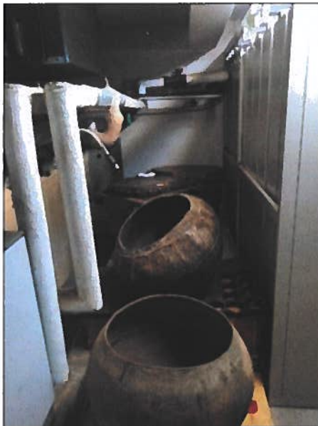
Figure 27: Objects stored directly below piping, exposing them to potential risks.
