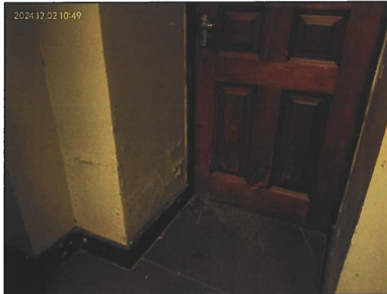
Figure 3: Visible damp on lower sections of walls.
