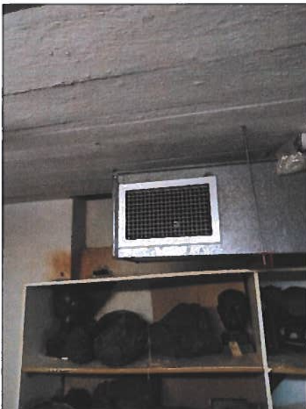
Figure 31: The only functional air-conditioning unit in the main storeroom.
