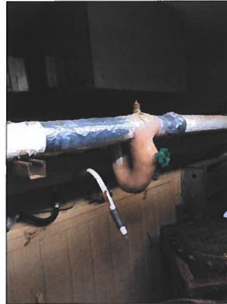
Figure 28: Patched pipes with artwork stored below.
